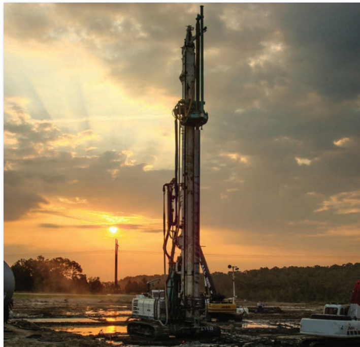
Soil mix columns constructed for foundation support and liquefaction mitigation for the expansion of a nuclear plant.
