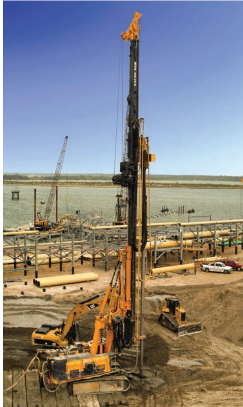
Soil mixing performed to increase bearing capacity and reduce settlement for planned tanks.
