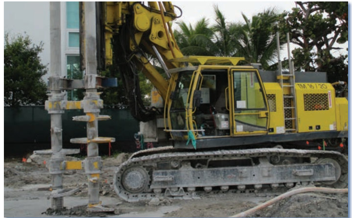
Dual axis wet soil mixing rig used to construct a perimeter retaining wall prior to excavation for a planned high-rise.
