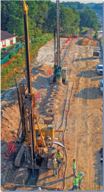
Above: Soil mix columns constructed along the alignment of an existing waterline provided a containment system to protect the critical utility.
