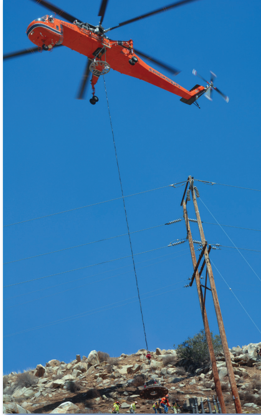
An example of our experience with a wide variety of applications—this remote, restricted access site for transmission lines required helicopters to mobilize equipment and materials.
