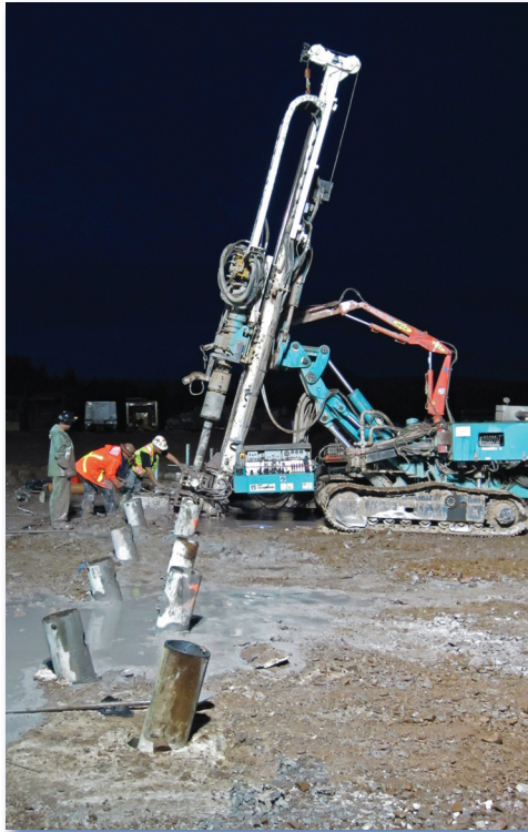
Installation of battered micropiles which can take both axial and lateral loading.
