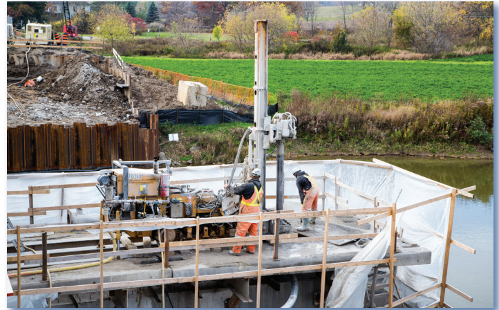
Small equipment being used to install micropiles through an existing bridge pier with a detailed spoil recovering system.
