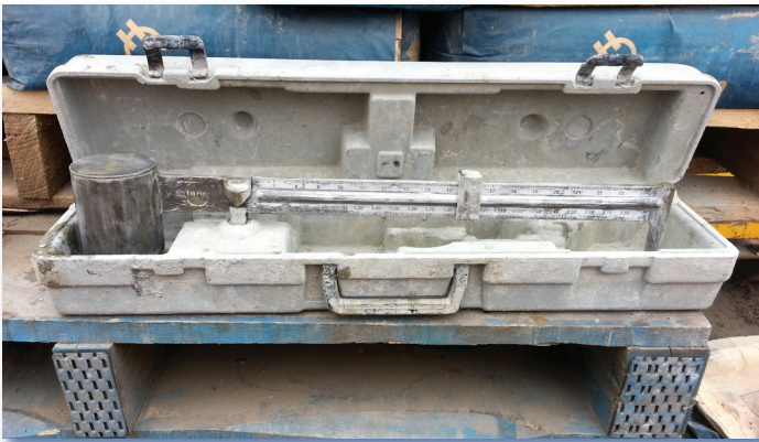
A detail QA/QC program is used with all Keller micropile installations. Photo showing mud balance being used to determine the specific gravity of the grout.
