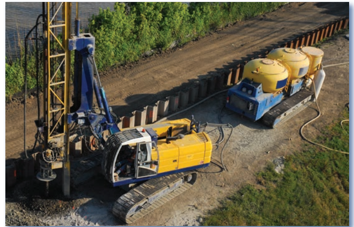
The accompanying shuttle supplies the binder, which is pneumatically conveyed to the binder outlet through the mixing tool system.
