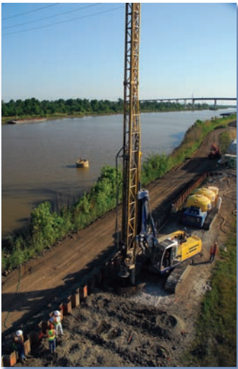
Above: Dry soil mix columns in shear panel arrangement being constructed from on top of a levee for ground improvement.
