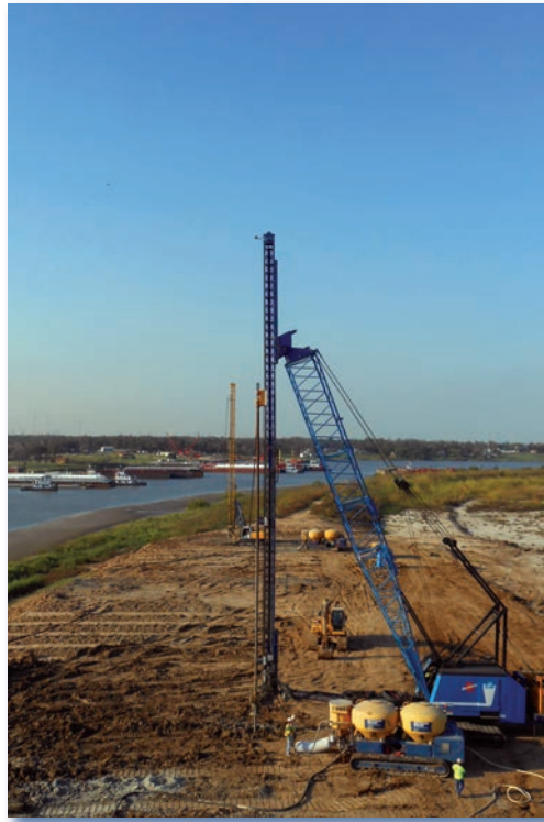
Dry soil mix columns to repair a levee failure on a dredge disposal island.
