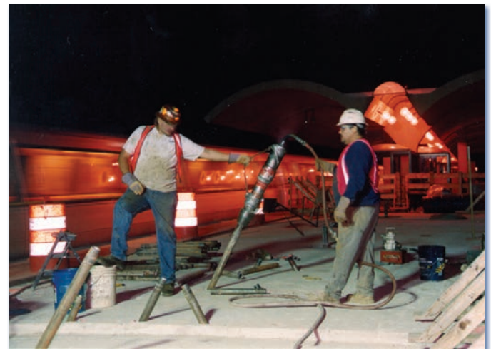
The Denver System of compaction grouting was used to consolidate fill beneath two, settling subway platforms.
