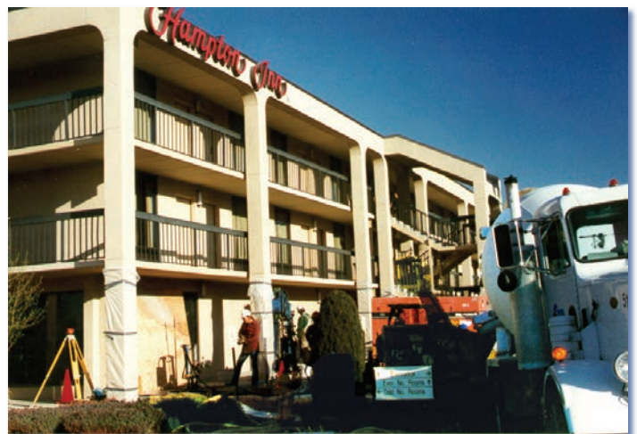
Remedial compaction grouting successfully treated collapsible soils beneath the hotel, reducing future settlement potential to an acceptable level.
